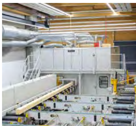
| In the new finish planing hall of Hördener Holzwerke.
